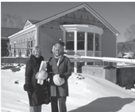
Board member Barbara O'Connell (left) and Program Committee member Ann Shriver Sargent admire the progress made on the construction of the Education Center.
