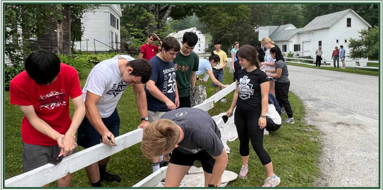
Coolidge Scholars sand and repaint the fences in the historic village in anticipation of the 4th of July celebrations.
